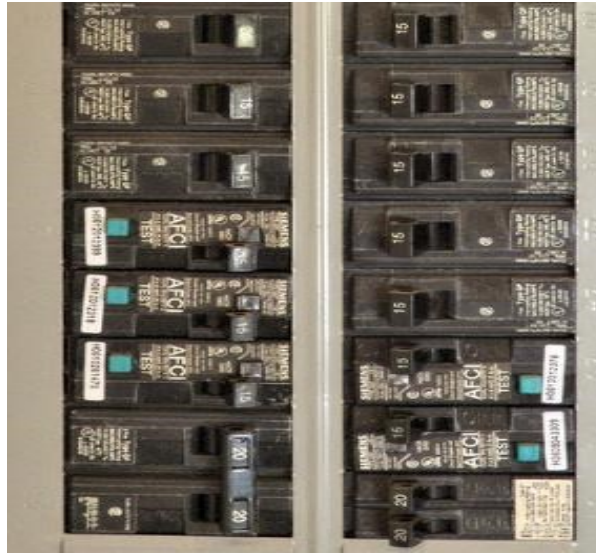
Figure 6. Breaker Box Equipped with GFI Breakers.
